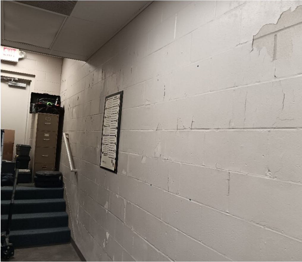
Existing concrete masonry unit walls have water damage leading to surface failures including some surface cracking as well as paint peeling from the surface.
