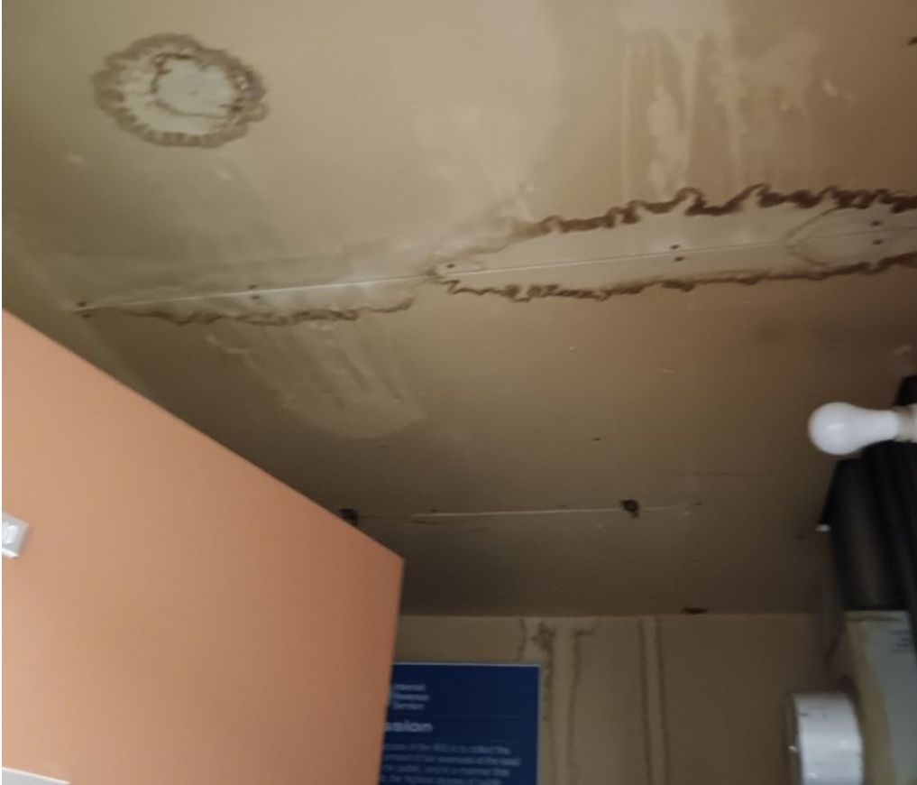
Drywall ceiling has extensive water damage. This is probably due to roof leaks in this area.
