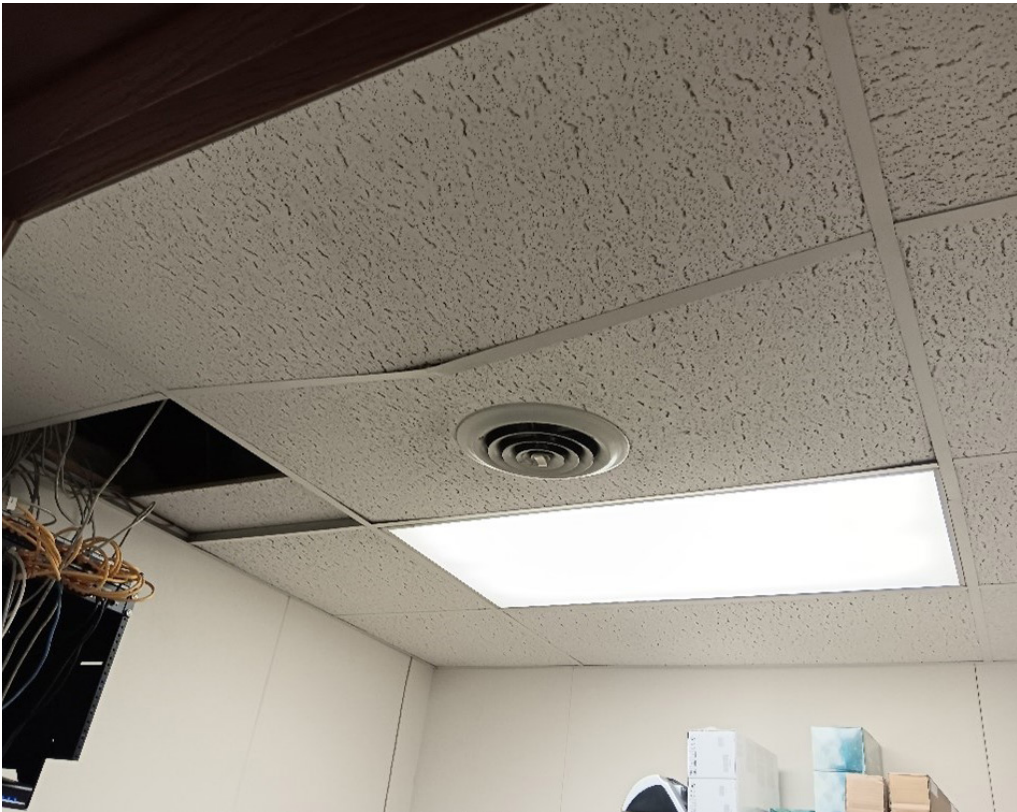
Ceiling grid systems are failing in various areas.
